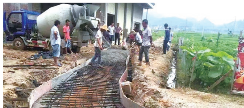
▲ Luoding Cement helped Fengtang Town to newly construct and repair cement roads
